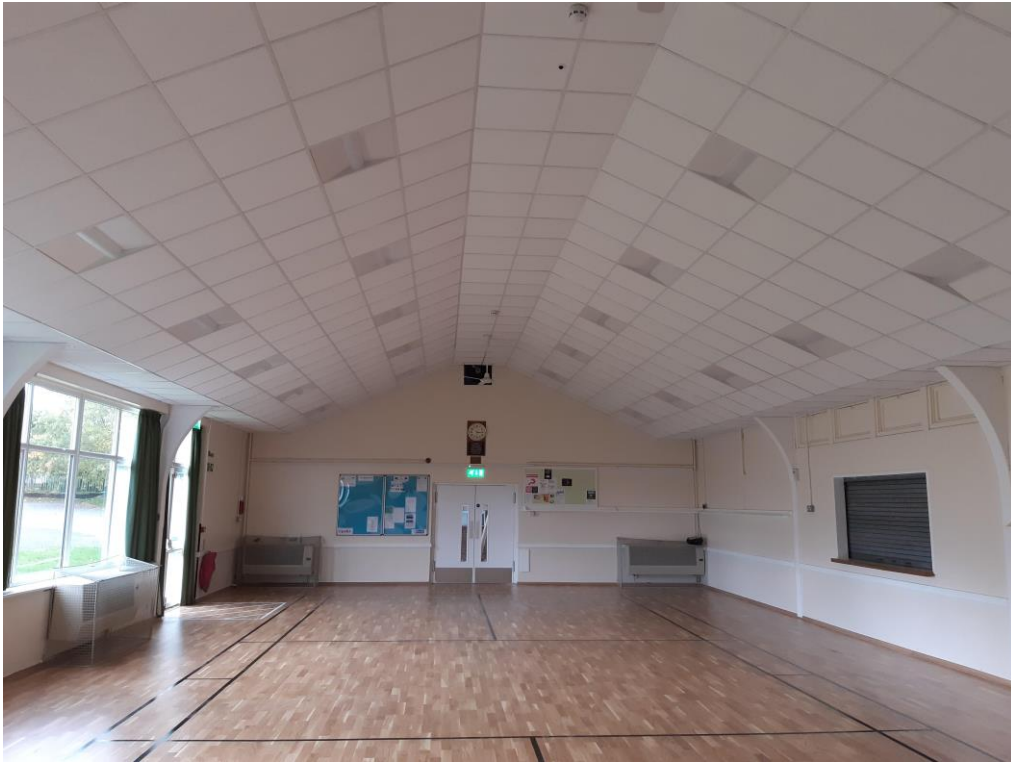
The main hall after completion of the new flooring, ceiling with integrated lights and emergency lighting, fire detection system and new fire doors with illuminated fire exit signs.
