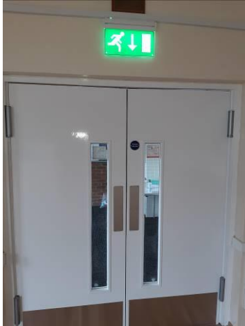
Picture shows new fire doors and illuminated emergency exit sign.
