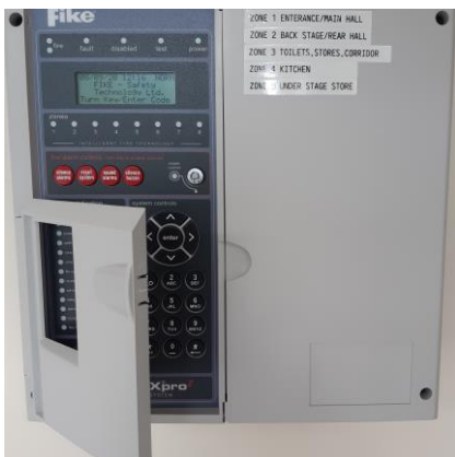
Main control Panel
