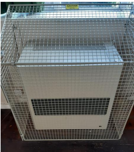
New back hall gas heaters
