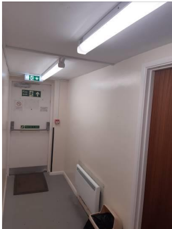
New lighting in the corridor with PIR sensors
